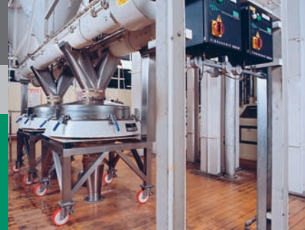
Compact 900 Sieves with Vibrasonic® deblinding system at Colmans - mustard powder producer. The screens are fed from blenders and pass the sieved material through to the packaging area.
