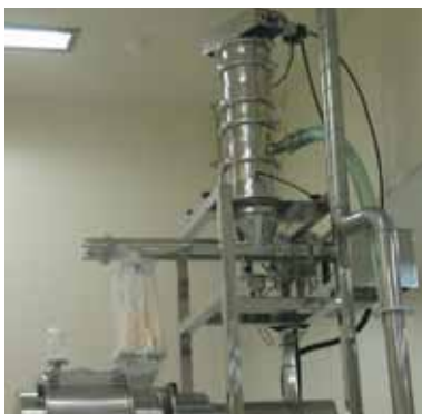
An example of Piab installation for powder transfer.
